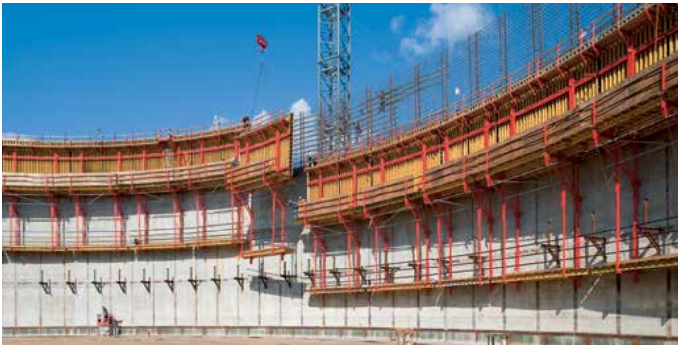
LNG liquid gas tanks Circular walls Ø 77.50 m with CB 240 and VARIO GT 24.
