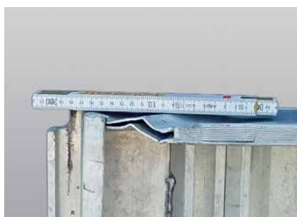
Stair Tower ■ deformation / damage at one point of the frame profile on the landing guardrail
